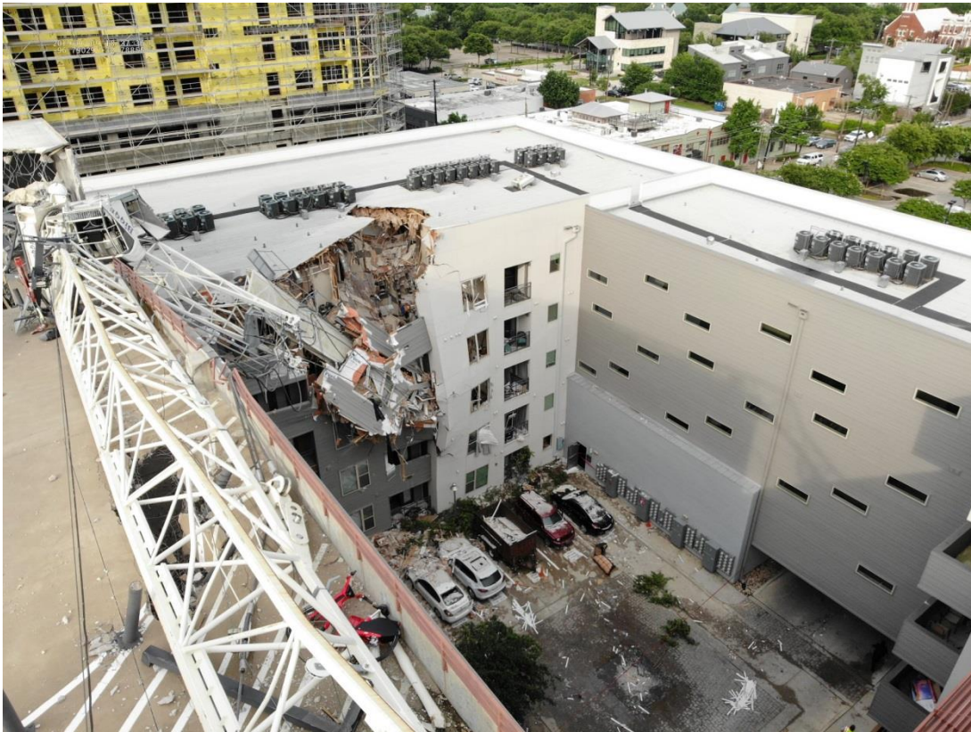
Photo Courtesy of North Texas PSURT team, two cranes collision
